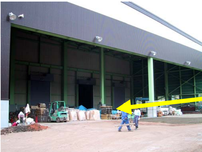
Platform and Pit door
