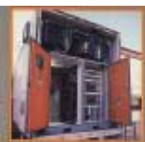
Power supply and auxiliary systems
