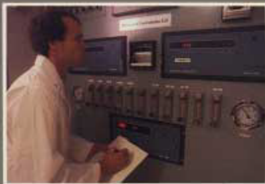
Gas monitoring equipment
