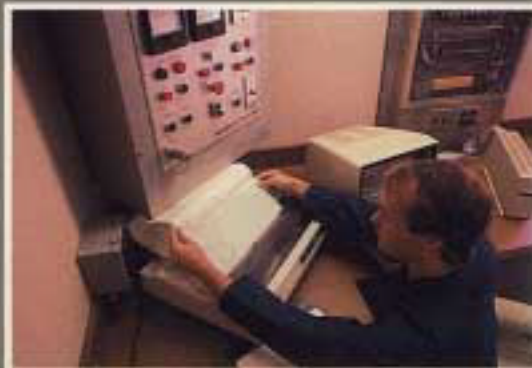
Gas monitoring equipment
